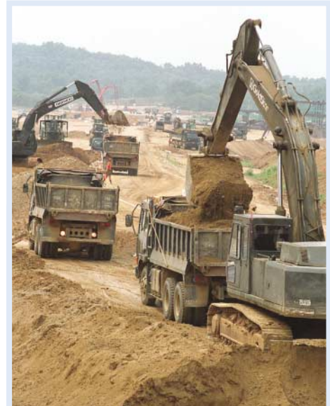
Roadbed construction work to reconnect the Gyeongui (Seoul-Sinuiju) inter-Korean railways and roads
